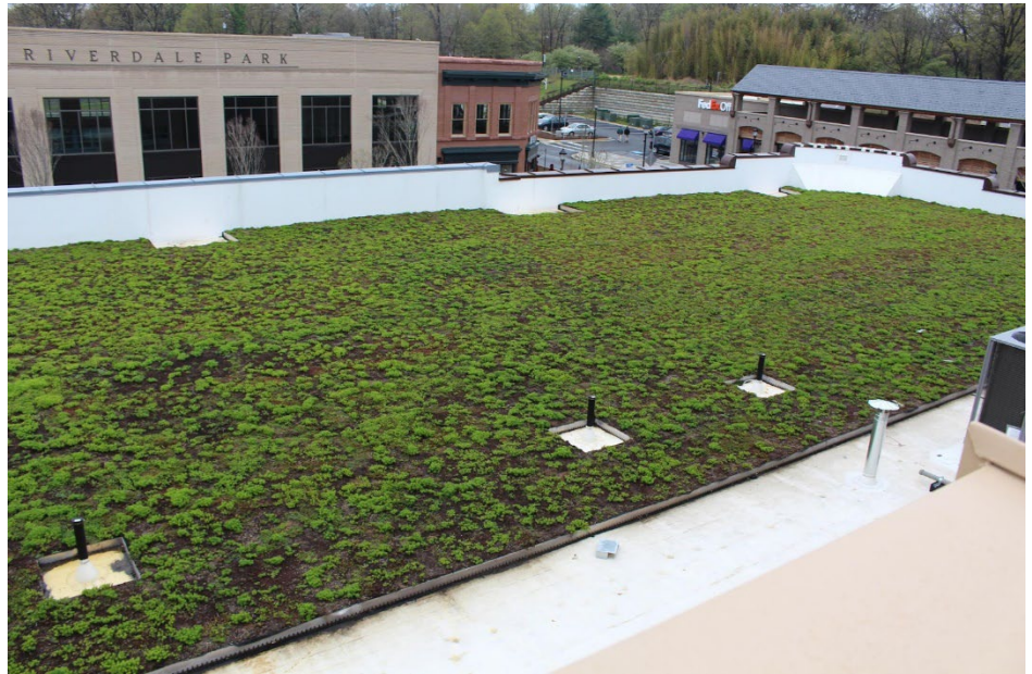
A green roof at Riverdale Park Station offers both stormwater management and pollinator habitat benefits.
